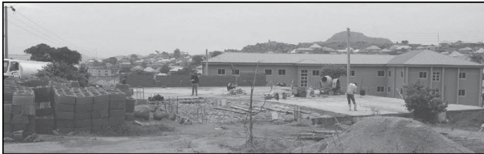
Looking north, the foundation and floor are now completed and the walls are going up!
